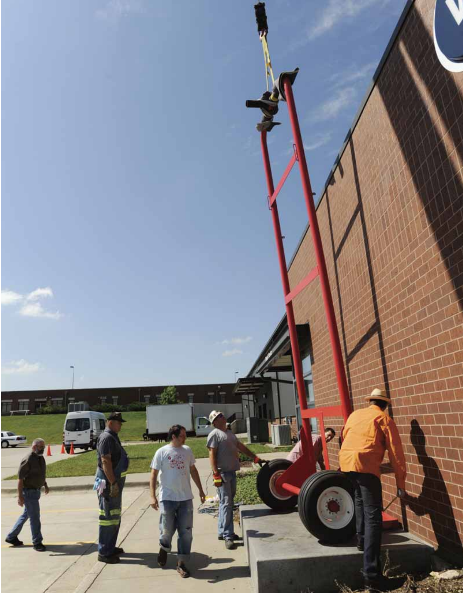
Artist Michael Schonoff (center, T-shirt) oversees the installation of his sculpture at the campus Warehouse.
