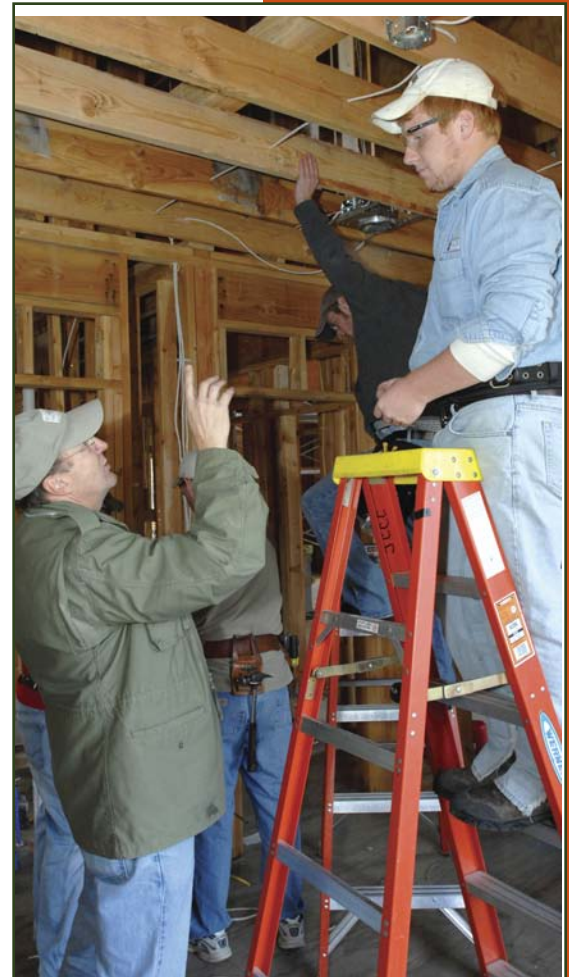
Mike Weible, professor, career program facilitator, electrical technology, instructs Ben Toplikar on the wiring of a ceiling box.
